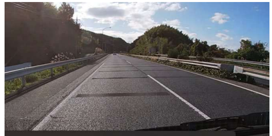
Fig.12 Condition of the road surface at point ②
