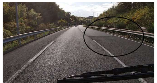
Fig.13 Condition of the road surface at point ③
