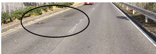
Fig.10 Condition of the road surface at point ①
