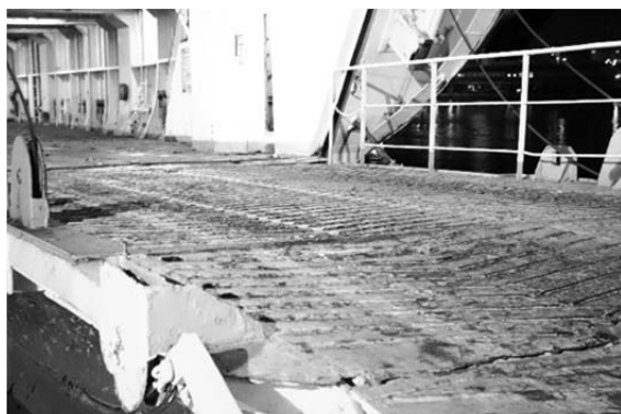
Fig.18 Unevenness of the rampway surface
