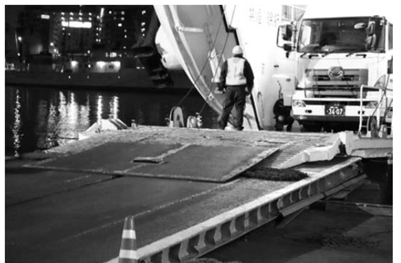
Fig.17 Step between the ramp way and the harbor road
